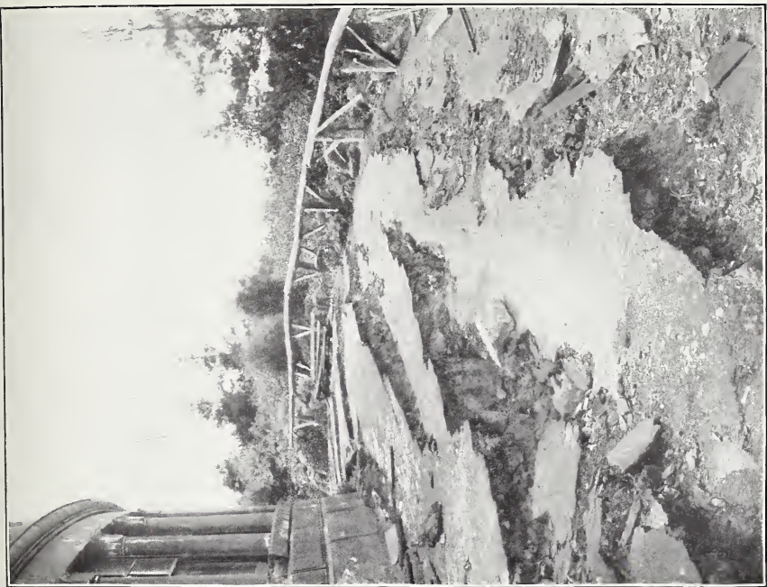
42. SLIP OF FOUNDATION OF CYCLORAMA, STRAWBERRY HILL, GOLDEN GATE PARK, SAN FRANCISCO, CAUSING COLLAPSE OF THE STRUCTURE.
